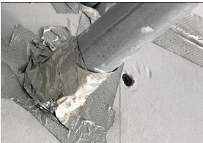
QuietRF® Shielding Tape around conduit
