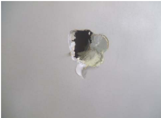
Figure 1: Damaged Gypsum Panel
